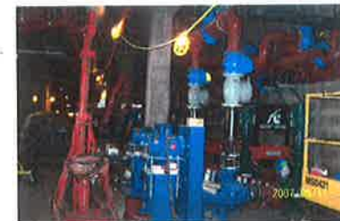
North area of pump gallery.
