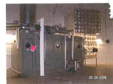
Heating and ventilation equipment.
