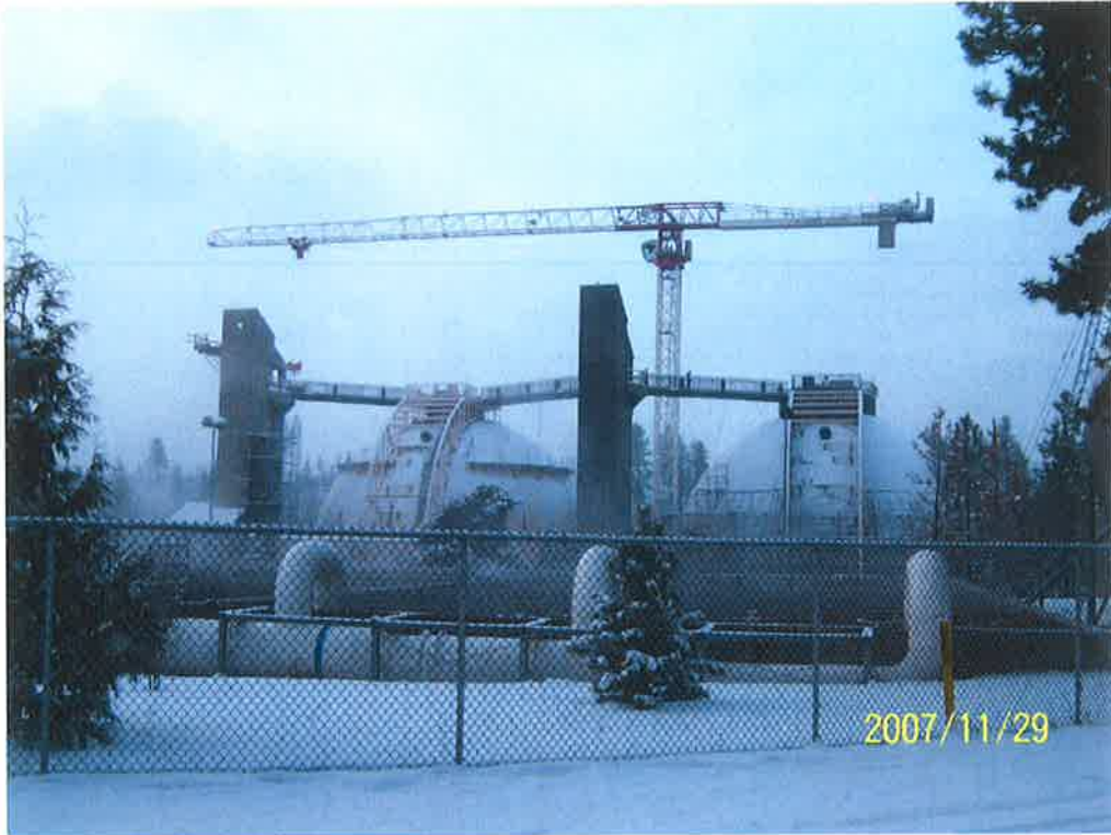
Exhibit I: Looking south to digesters, winter of 2007.
