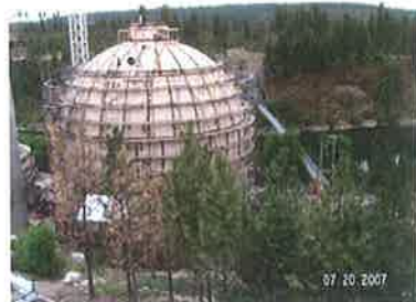
Egg-shaped digester, Riverside Park Water Reclamation Facility.
