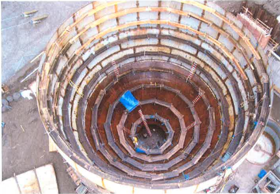
Exhibit E: View of inside of digester from crane.
