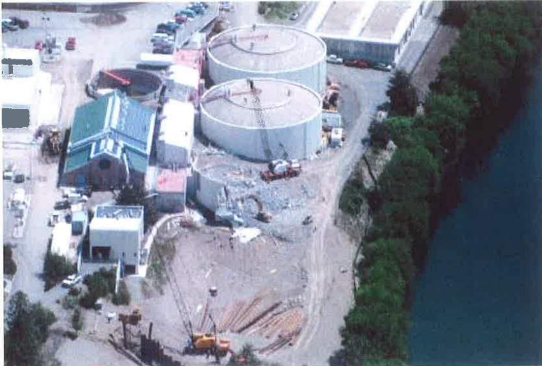
Exhibit A: New boiler building at upper left (green roof), old boiler building to south, and Digester 3 demolition (center).
