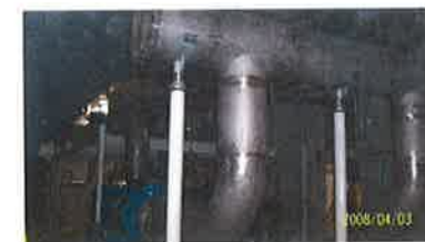
Digester mix piping.
