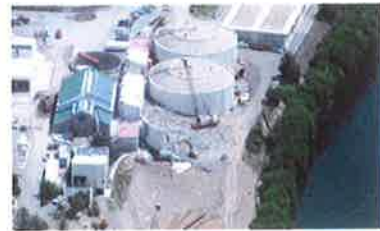
New power building upper left (with green roof), old boiler building to south, Digester 3 demolition (upper center.)
